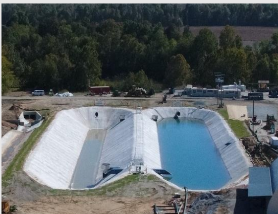
Process Water Basins
