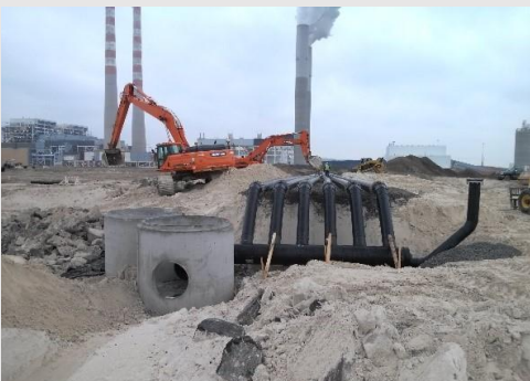
Header and Valve System
